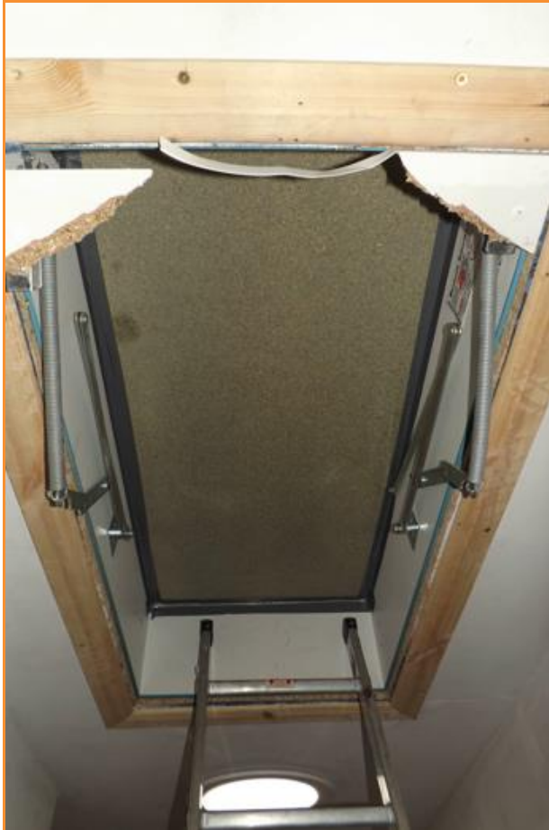
8.04: Leakage around the edges of large loft hatch – temporarily sealed to quantify by subtraction the significance of the problem.
